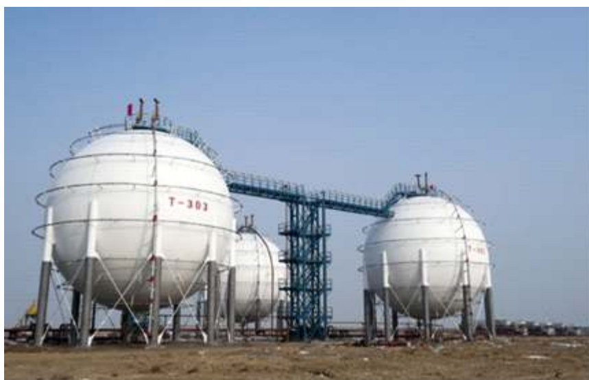
A petrochemical plant owned by Alashankou Horizon Petroleum and Gas Inc. seen at Alashankou Comprehensive Bonded Zone in Xinjiang Uygur Autonomous Region.
